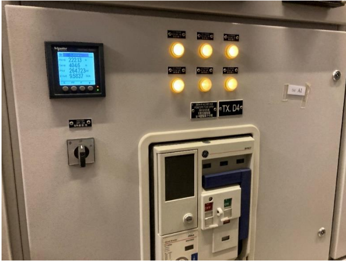
Switchboard and Power analyzer
