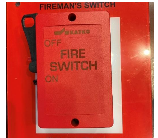
Fireman's emergency switch
