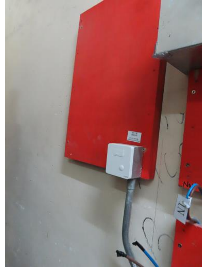
Meter board for power company's Tariff Meter Communication (TMC) Infrastructure
