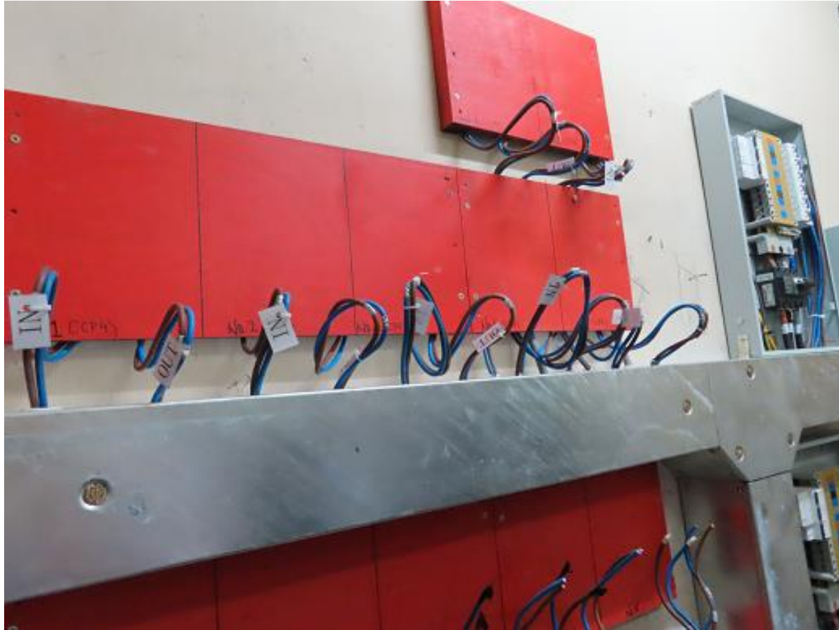
Meter boards for power company's electric meters
